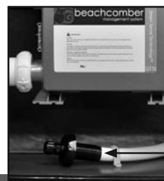
Drain / Fill Valve
